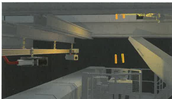
The Gob Master consists of two high speed cameras, a control unit, a water chiller and a monitor.
